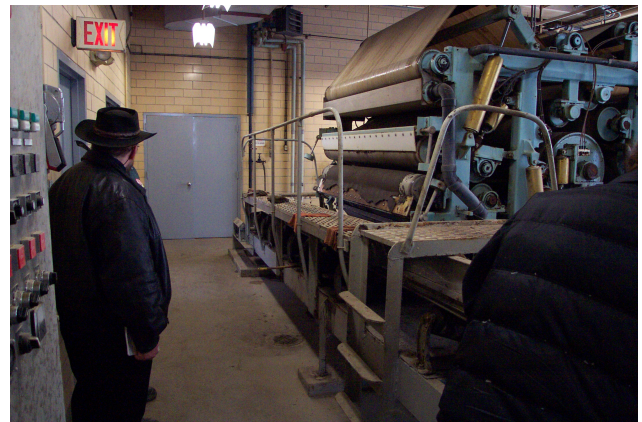
Dewatering wastewater solids (sludge) with a belt filter press.
