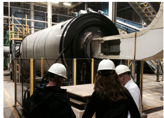
Rotary-drum heat drying of biosolids at Greater Lawrence Sanitary District
